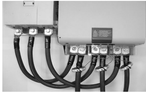
Figure 9.15 - CTs to external current acquisition
